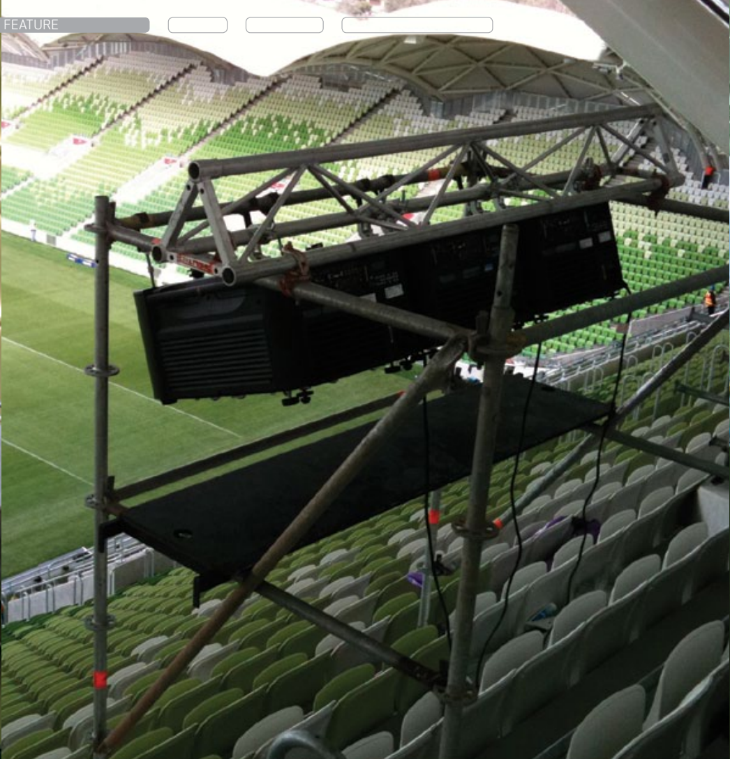
One of the six clusters of Christie Roadster S+20K projectors that had to be mounted on scaffold towers above the seating when it was discovered that the roof was not load-bearing.
