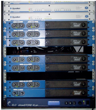
One of the zoned equipment racks with Powersoft amplifiers and Symnet Express DSP processors
