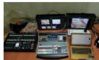
A/V control systems for the main sanctuary
