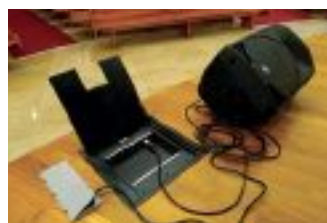
Self powered Mackie SRM350 floor monitors can be connected to any of the five facility panels on stage
